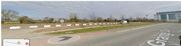
Building of a berm at Grange Castle, South County Dublin, with temporary Kelly Blocks in the background
